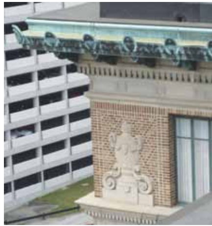
The copper cornice and finial design were added to the building in 1932. The preservation work that was done in 2003 included replacing a damaged section of the cornice with copper aged to match the original.
