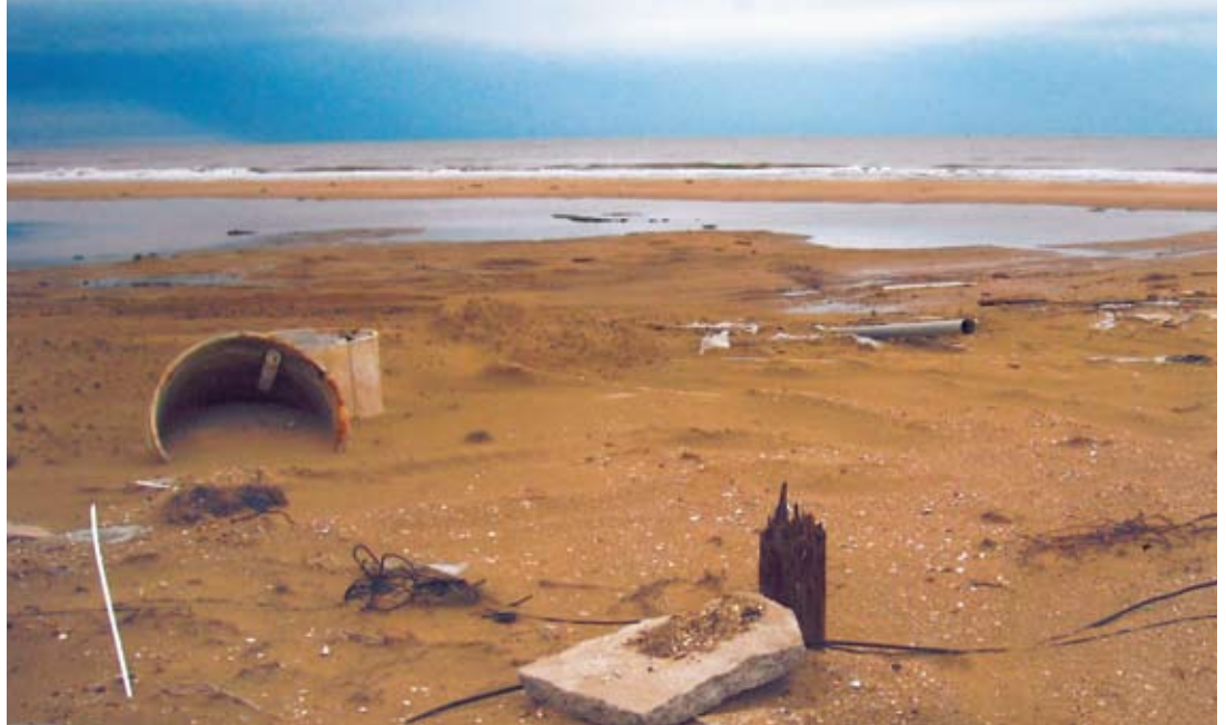
The view from under the late deck of the Murphy house after Ike.
