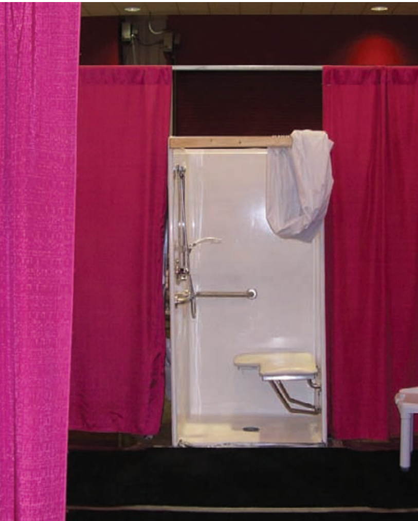
The City of Houston successfully installed showers, washing machines, and sinks in order to ensure sanitation in the shelters.
