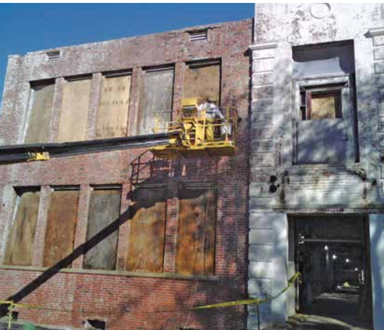
After years of neglect, restoration of the 1926 structure began in late 2008. Power washing the exterior to reveal the original brick surface was a top priority. Structural damage to the building is visible on the top-left corner. Also apparent is the dismal condition of the interior.
