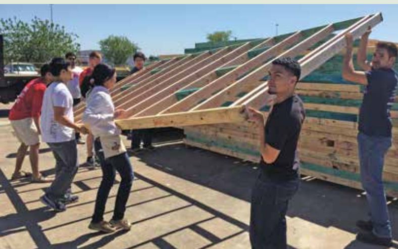
The University of Houston Habitat for Humanity Campus Chapter members work to assemble a new home.
