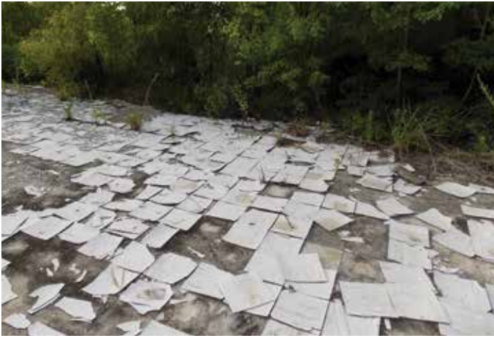
This foundation, located on MacArthur Avenue, still contains remnants of red carpet, white linoleum tiles, and red bricks.
