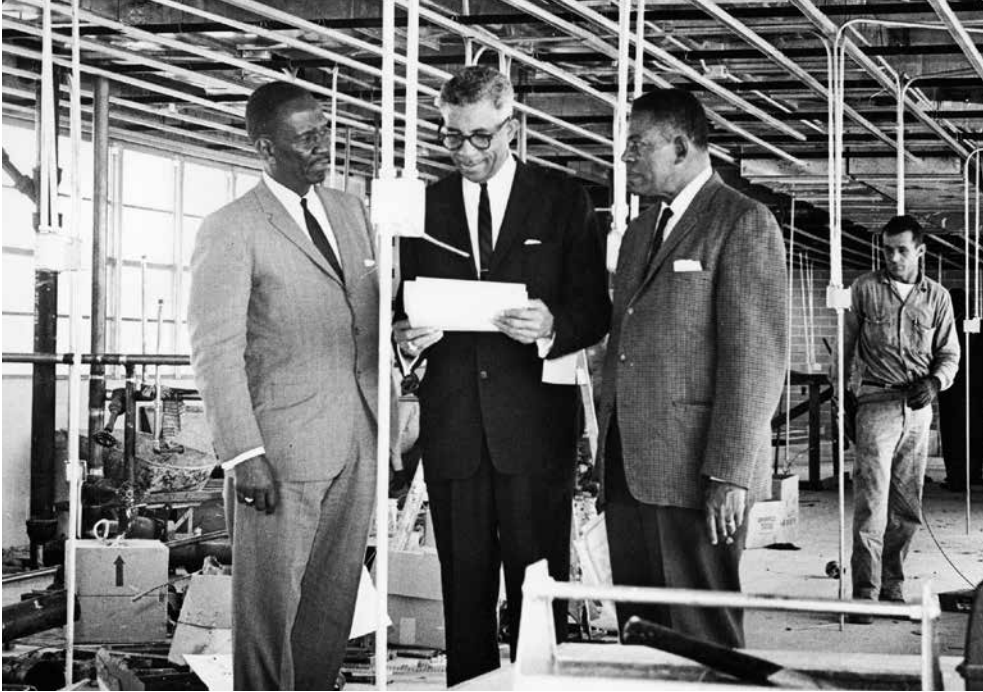
Judson Robinson Sr. (center) and two other men check on construction at the YMCA in Southeast Houston.
