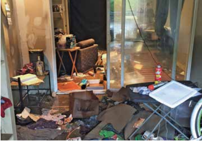
The damage was extreme, with four feet of water inside, drenching even what had been elevated on a platform. The roof also collapsed in multiple places. The foul, murky water that flowed throughout the building's ten units smelled of sewage and left an oily film on everything it touched.
