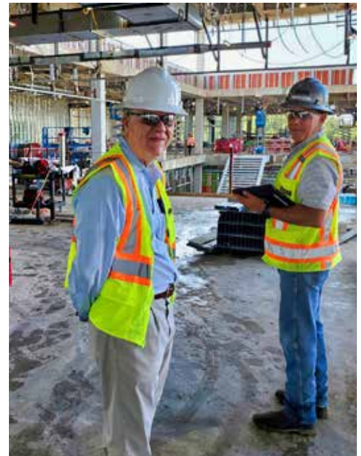
Dean Stephen Spann, left, visits the UH College of Medicine construction site.
