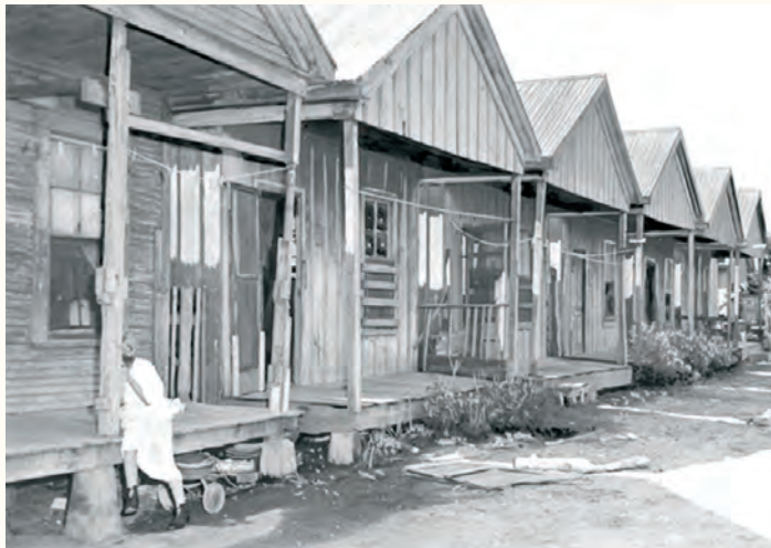
Residents of the El Alacrán barrio, known originally as Schrimpf's Field, dealt with dilapidated housing conditions following the departure of the area's early German residents.
